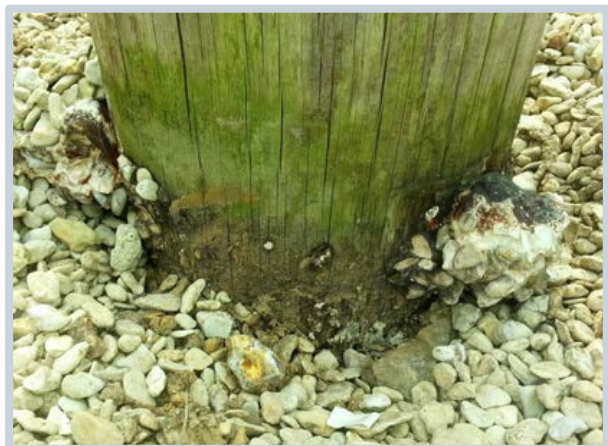
Scrap away the gravel and fungal growth on the pole can be seen and should be done according to the manufacturer's or supplier's instructions for maintenance.
